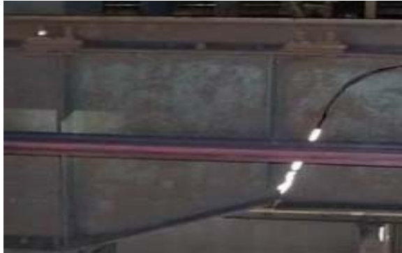
Fig. 10. The actual cracks of trapezoidal variable cross-section crane girder.
