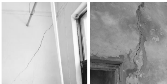
Fig. 1. Crack of wall in houses.
