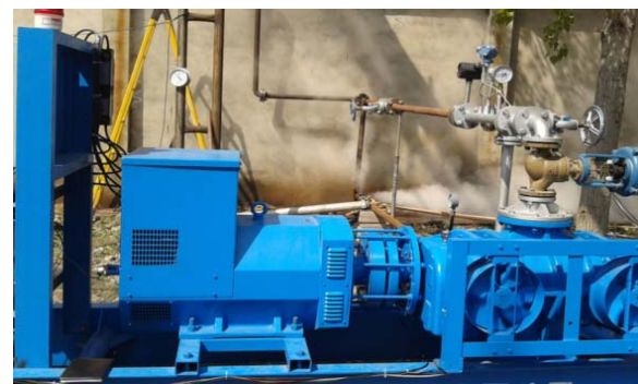
Fig. 3. The photo of Roots-steam generator.
