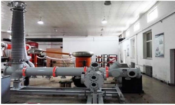
Fig. 9. The 252 kV GIS PD experimental platform.
