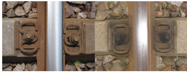
Fig. 3. Fastener Image Samples of natural corrosion and environmental interference.
