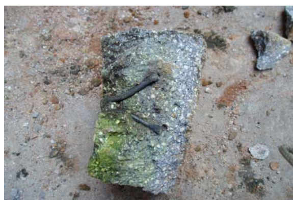
Fig. 4. The detached castable and anchors.
