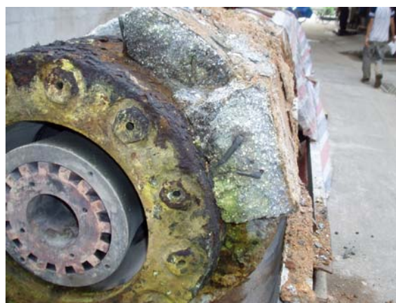
Fig. 3. Damage of the end.
