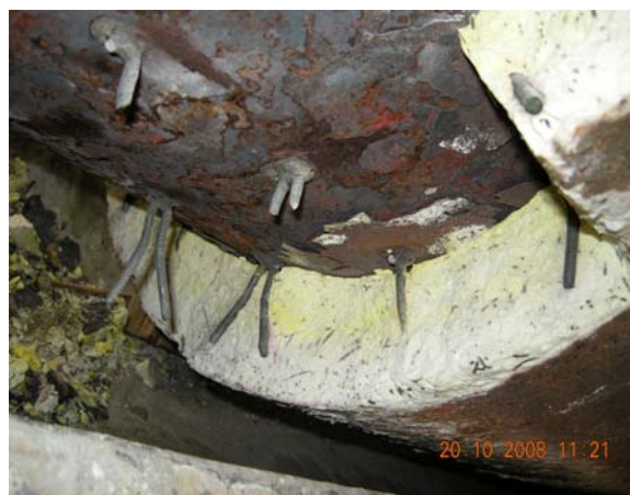
Fig. 2. Castable and anchor detach from the burner.
