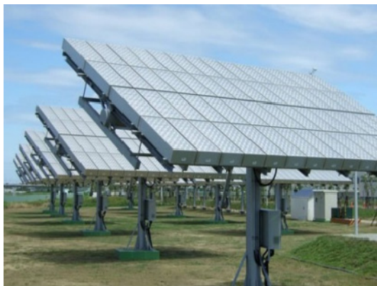
Fig. 2. Solar power station.
